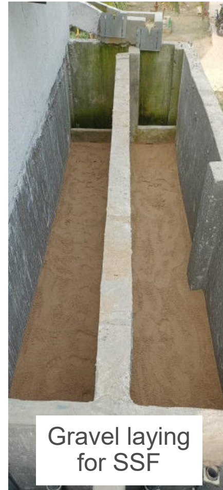
Gravel base in SSF
