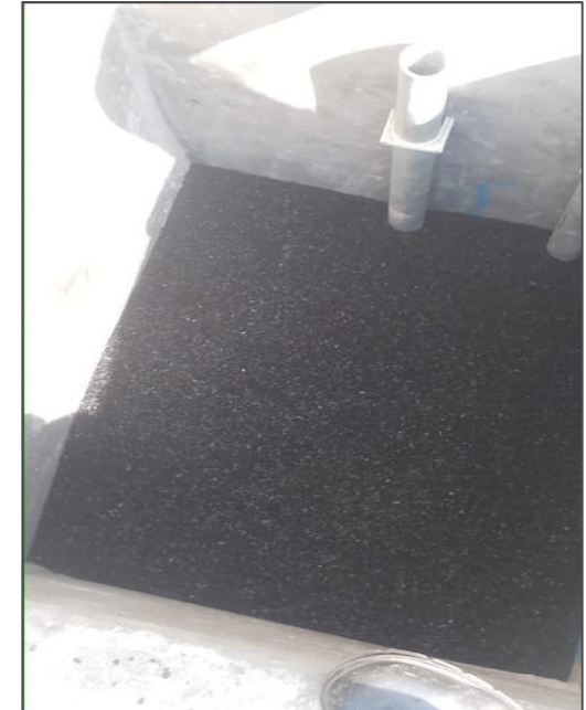
Activated Carbon Media filling
